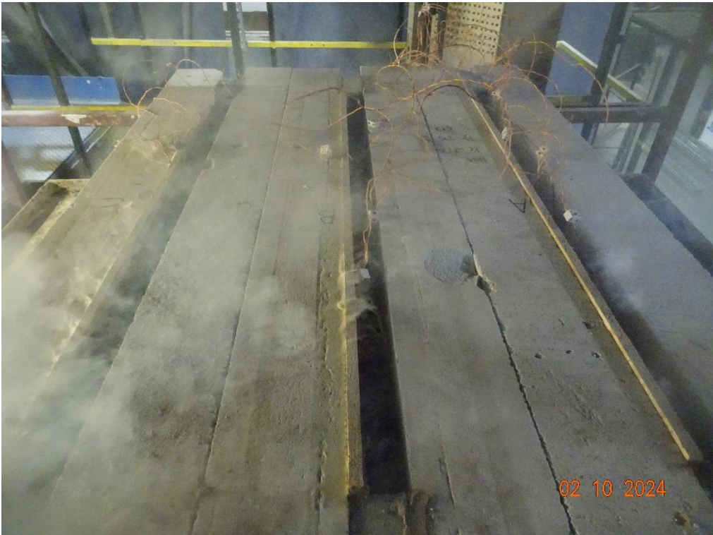
The unexposed face of the floor assembly after a test duration of 30 minutes
