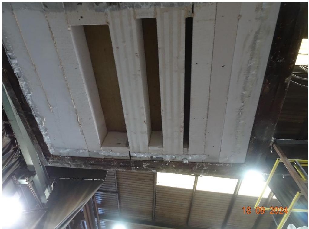
The exposed face of the floor assembly immediately after the test duration
